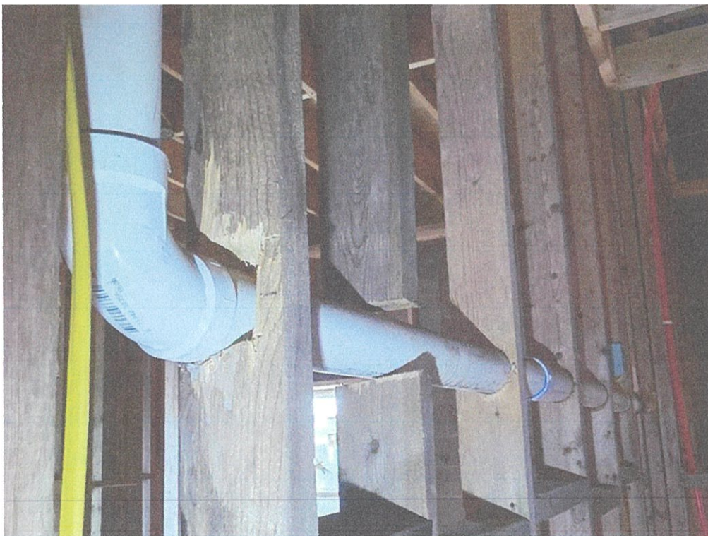
2x4 wall cut in half or missing more than 50% of its volume.
