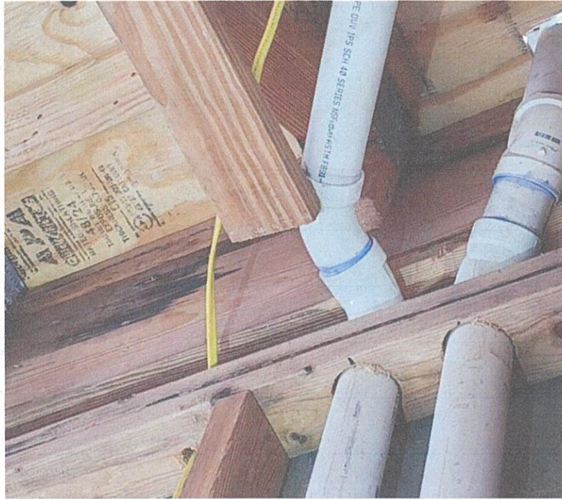
Cut truss end in between 1 st and 2 nd floor at left side of residence.
