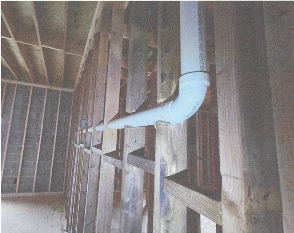
2x4 wall cut in half or missing more than 50% of its volume.
